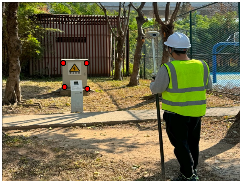
Hazardous location- Electricity Site
